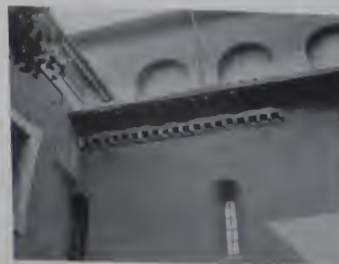
Fig. 74. S. Maria. East part of aisle wall. Brick construction of anteroptic masonry, masonry and joints, cornice, ledges.
